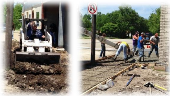
Melvorn PRIDE members prepare to replace sidewalk for the Melvorn Community Center
